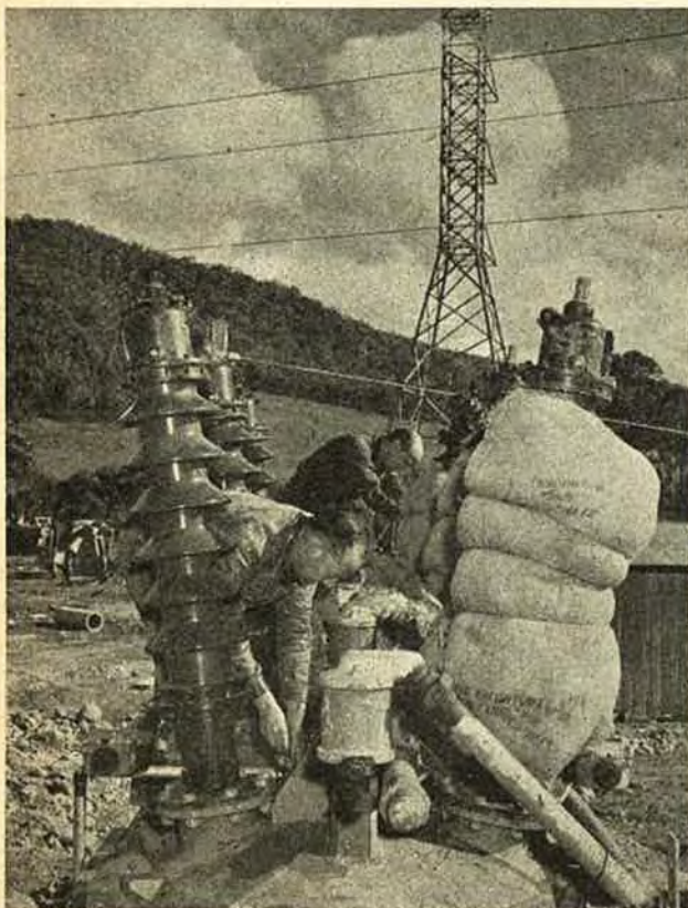
Installing 66 kVA oil circuit breaker at Mt. Beauty. Insulators are wrapped in bags to protect them in transit
