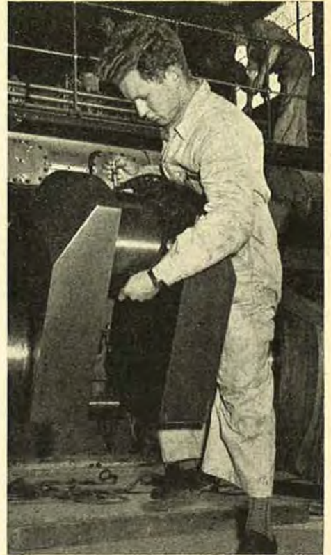
Engineer Graham Hoinville rides the crankshaft of the new diesel generating set at Shepparton power station.
