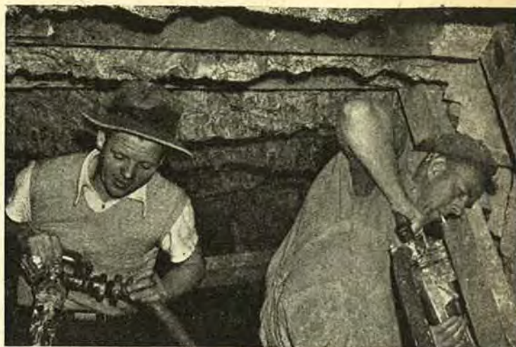
Working beneath Russell Place, "Snowy" Coyle and Joe Downs are making excavations for a new underground main feeding a City Council sub-station.
